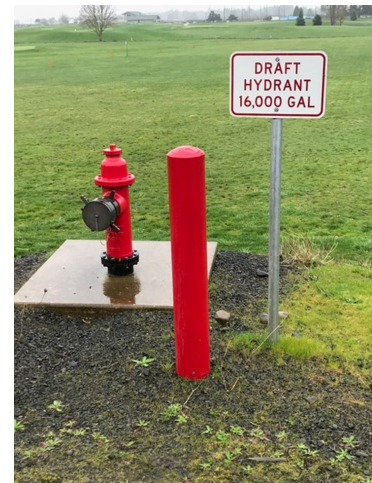
Limited supply hydrant
